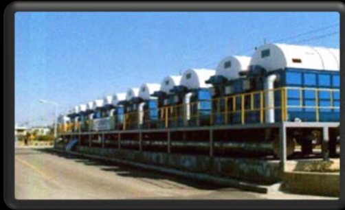
State of the art Sewage Treatment plant
