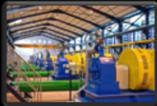
Water treatment for potable water
